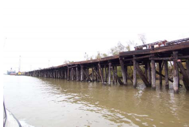
Damaged wharfs along Mississippi
